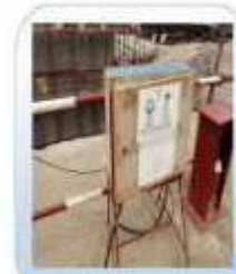
Electrical panel board (power) open condition. Electrical panel boards to be closed and left at all times. Only authorized electrical personnel are to operate.
