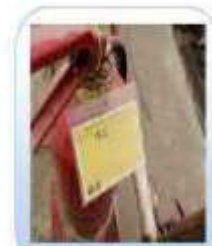
Blocked fire extinguisher fire hose. Fire extinguisher must be inspected and ready for immediate action by competent person.
