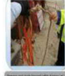
Storage and single (Storage) safety harness not used.
