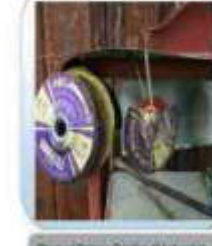
Personnel (Personnel) not wearing safety harness.
