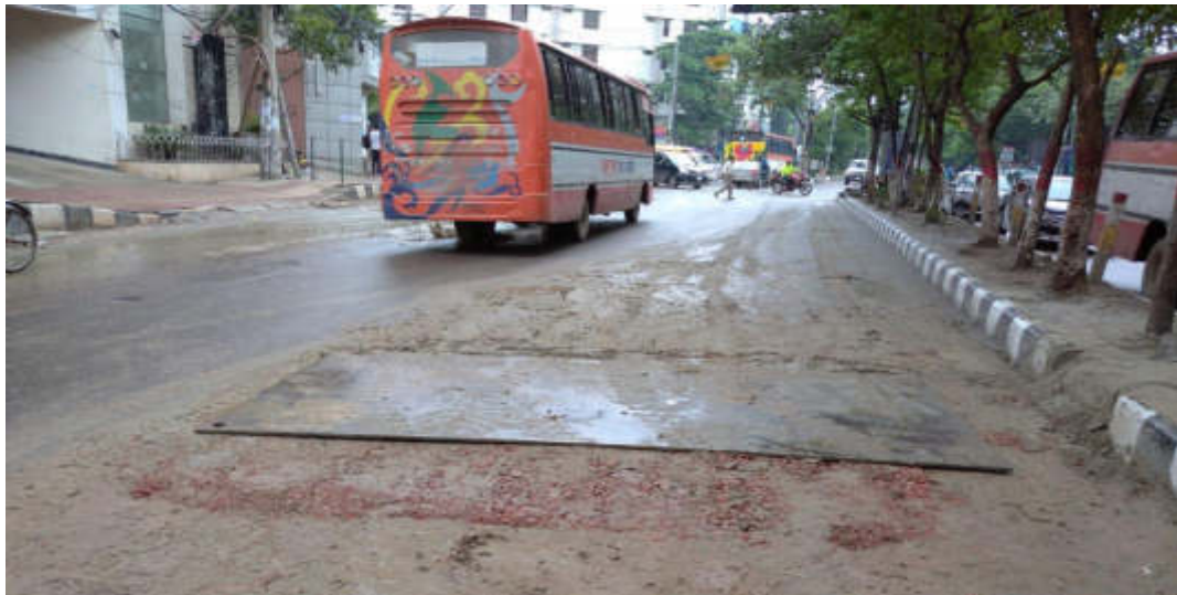
Steel sheet are in use to facilitate traffic movement at Shahjahanpur rd crossing DMA 615 on ,13.06.20
