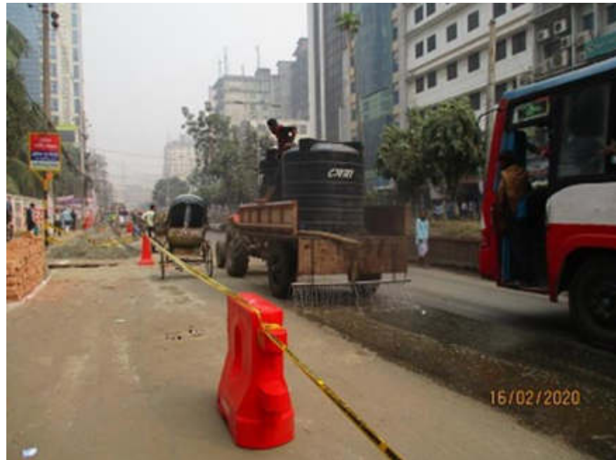
Water spraying to reduce the dust at the work site of DIT road at DMA 616
