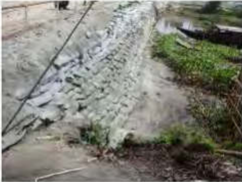
Sand fill in adjacent land need to remove
